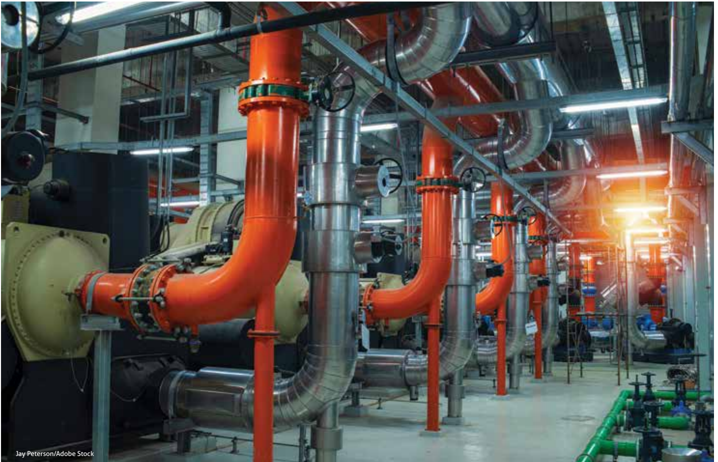
To constrain costs, upgrades like those shown here can be incorporated over time through a strategic utility master plan that ensures changes align with facility growth (or contraction) plans.
